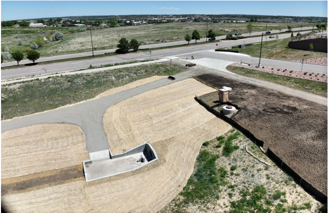
Figure 5:Constructed Forebay at the Downstream end of the project– Courtesy of SEMSWA
