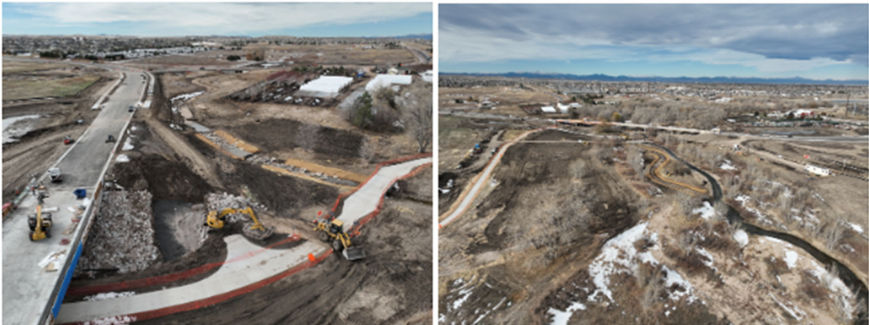
Figure 12. Construction progress photos of the Cherry Creek at Dransfeldt project (Courtesy of Mueller Engineering, November 2024)
