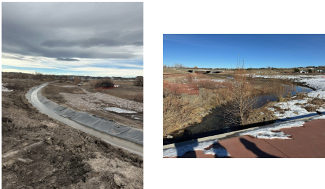
Figure 14. Construction progress photos of the Cherry Creek at Scott Avenue project (Courtesy of Mueller Engineering, November, 2024)
