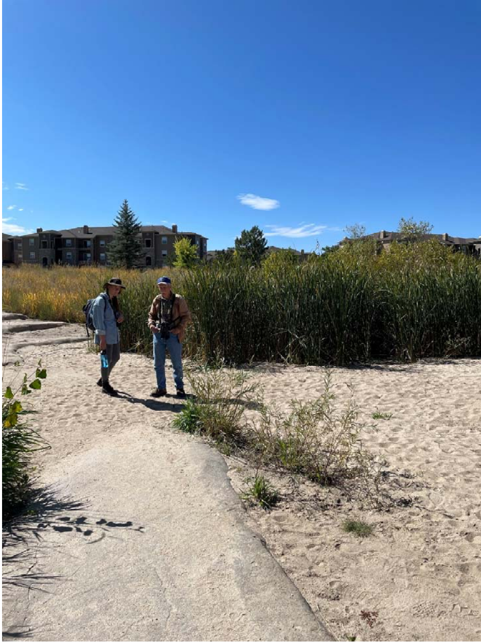
This photo shows sand that filled in the secondary channel that is part of the 'splitter drop' at Cherry Creek Valley Ecological Park. June, 2023
